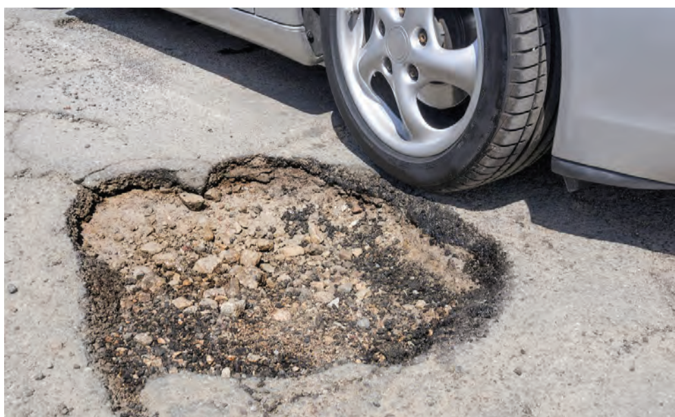
Potholes on roads a concern.
